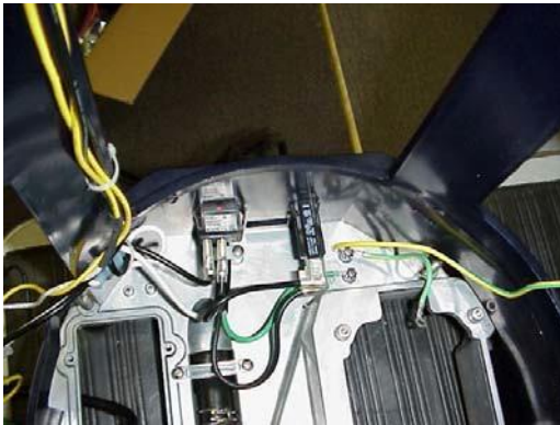
Figure 19. Power switch and circuit breaker.
