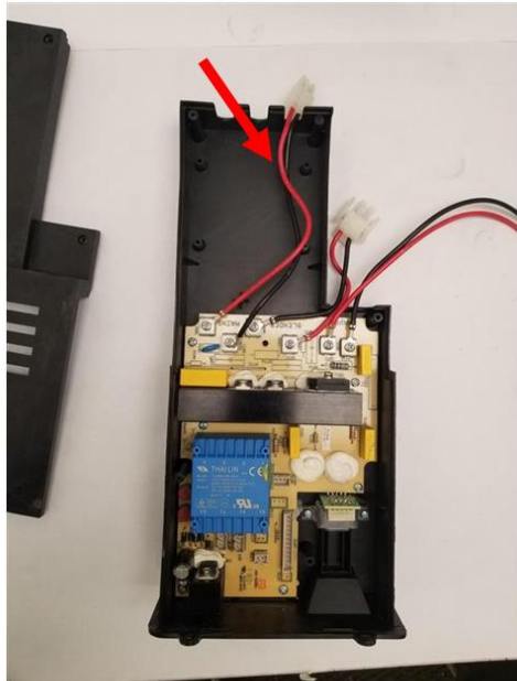
Picture of INCORRECT WIRING
