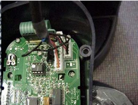
Figure 6. Wiring harnesses on rear of panel. Hold down removed for clarity
